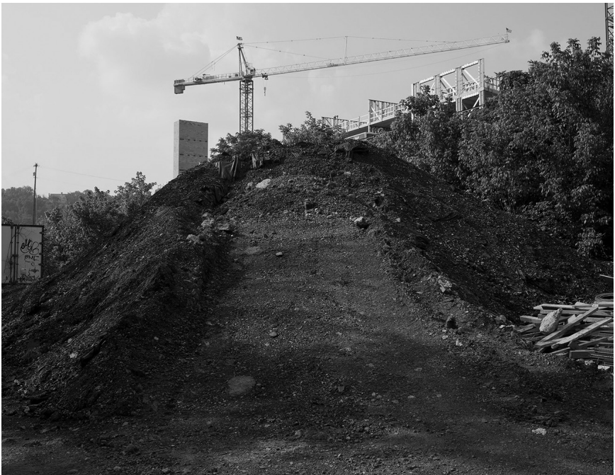
Image taken by activist George S. Bedell of all that remained of the main building at the Beaumont Glass Company after its demolition in 1998. Photo courtesy of George S. Bedell.
